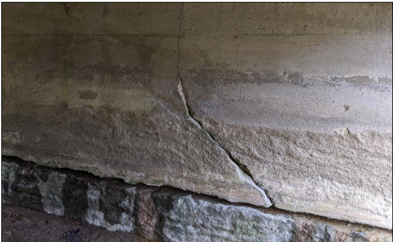
Figure 3. Sinclair Line over Nesbitt Drain – Wide Vertical Cracking on Culvert Walls / Footing Joint Separation
