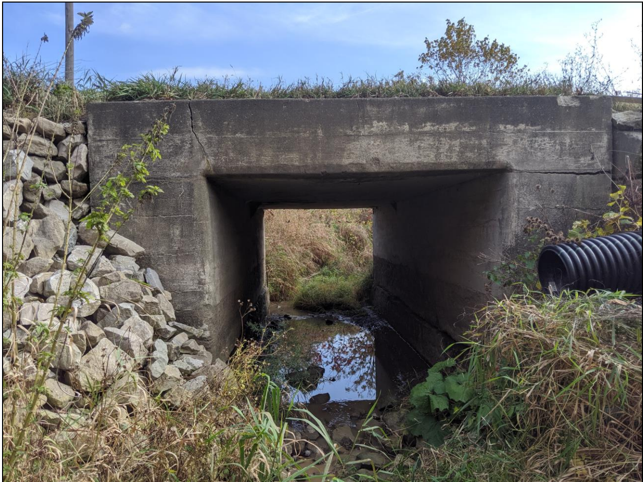
Figure 1. Sinclair Line over Nesbitt Drain – North Culvert End with Movement Cracking
