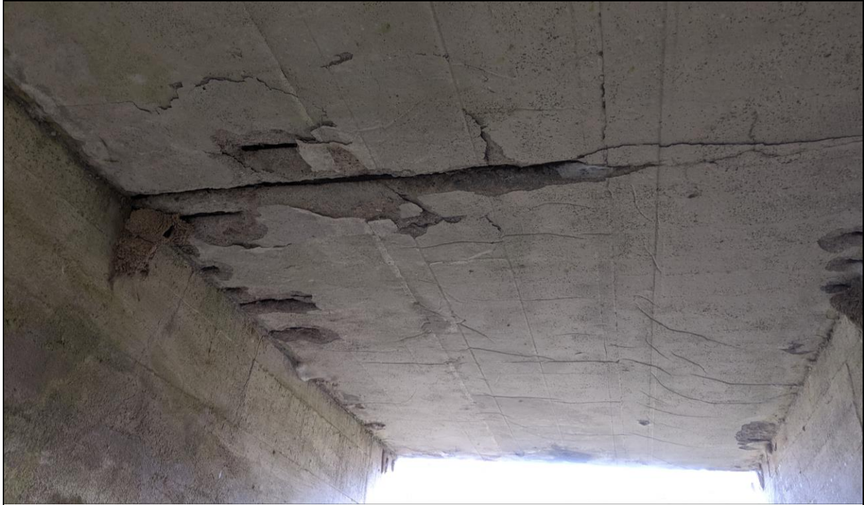
Figure 2. Sinclair Line over Nesbitt Drain – Soffit with Delamination and Spalling with Exposed Rebar
