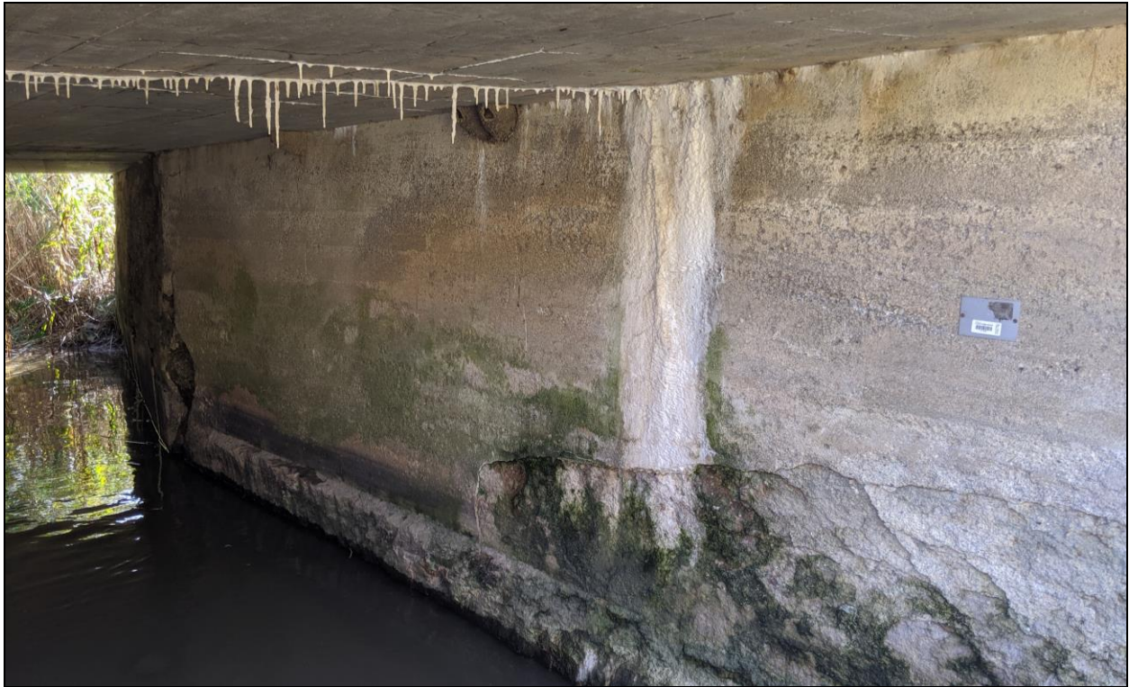
Figure 2. McKay's Line over Fields Creek Drain – Interior Barrel with Deterioration, Wide Cracking, Severe Spalling, Efflorescence, and Exposed Footings
