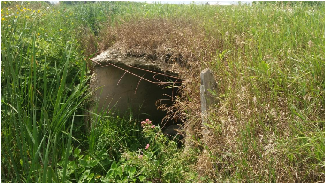
Figure 2. Union Line over Pollock Drain – South Culvert End Deterioration with Exposed Rebar
