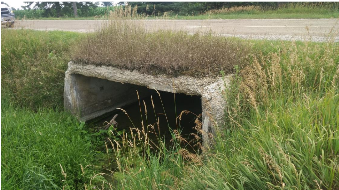
Figure 3. Pioneer Line over Forsyth Drain – North Culvert End Concrete Deterioration
