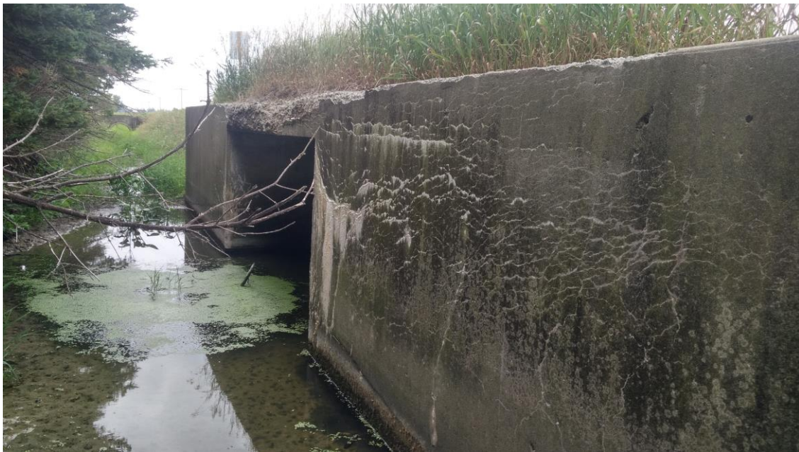
Figure 4. Pioneer Line over Forsyth Drain – South Retaining Wall with Cracking and Efflorescence
