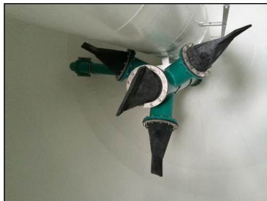
New internal water mixing system
