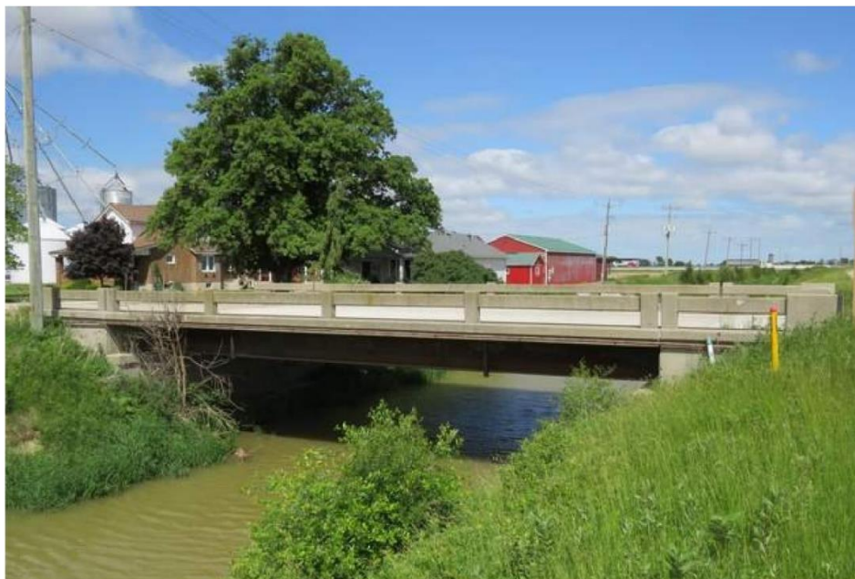
Figure 2. Gleeson Line over Government Drain #1
