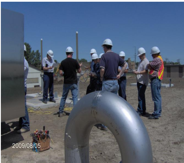
(Commissioning and Training of Staff at the Wallaceburg Water Treatment Plant)
